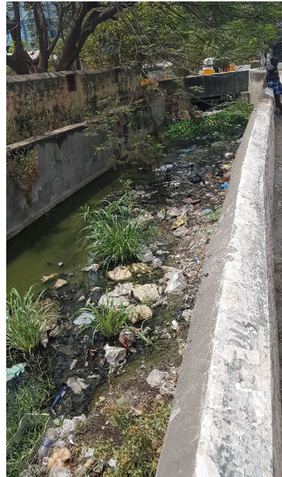
Figure 2: Clogged drains near Selvachintamani Lake in April 2022. Source: AQUA-Hub Project Team (Beckett)
